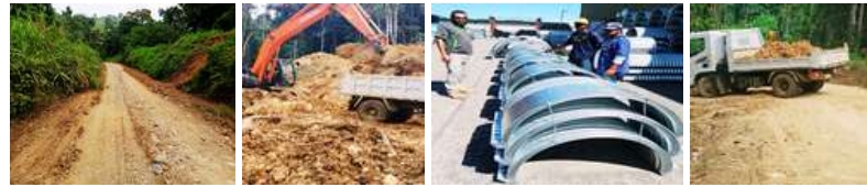
Below: Photographs of road works to provide accessibility to resettled Manam Islanders in Andarum, Madang. The completion of the pilot access road from Bogja to Andarum in 2023 is a major achievement under the Resettlement Infrastructure/Land-work component of the government's response.
